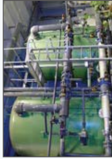
Environmental protection equipment
